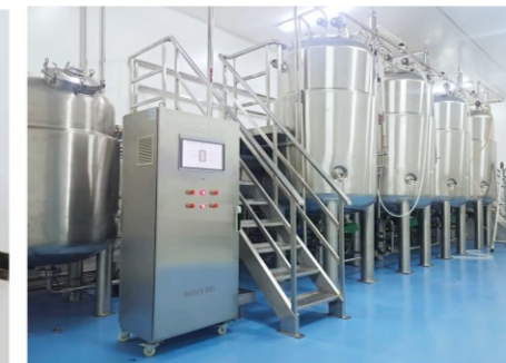
Four-tank inactivation system
